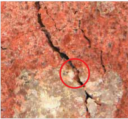
Crack formation in the concrete surface
