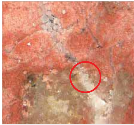
Crack healing by auto-reactive function in the concrete
