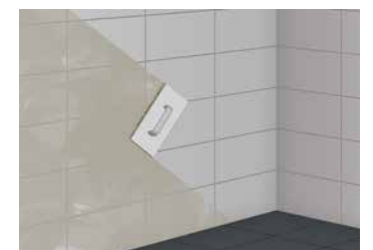
Note: The adjacent floor jointing process is also valid for wall areas
