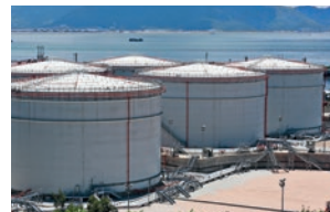
Tanks and containers
