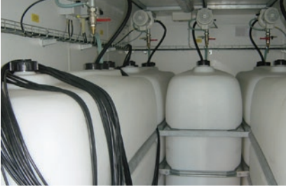
Storage and dosing of liquid concrete admixtures in the concrete plant (photo credit: Würschum GmbH)
